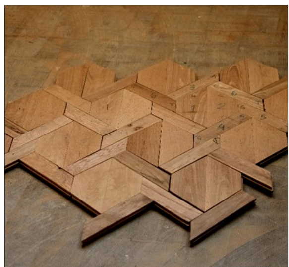
White oak parquet flooring with walnut edge banding and brass inlay under construction
